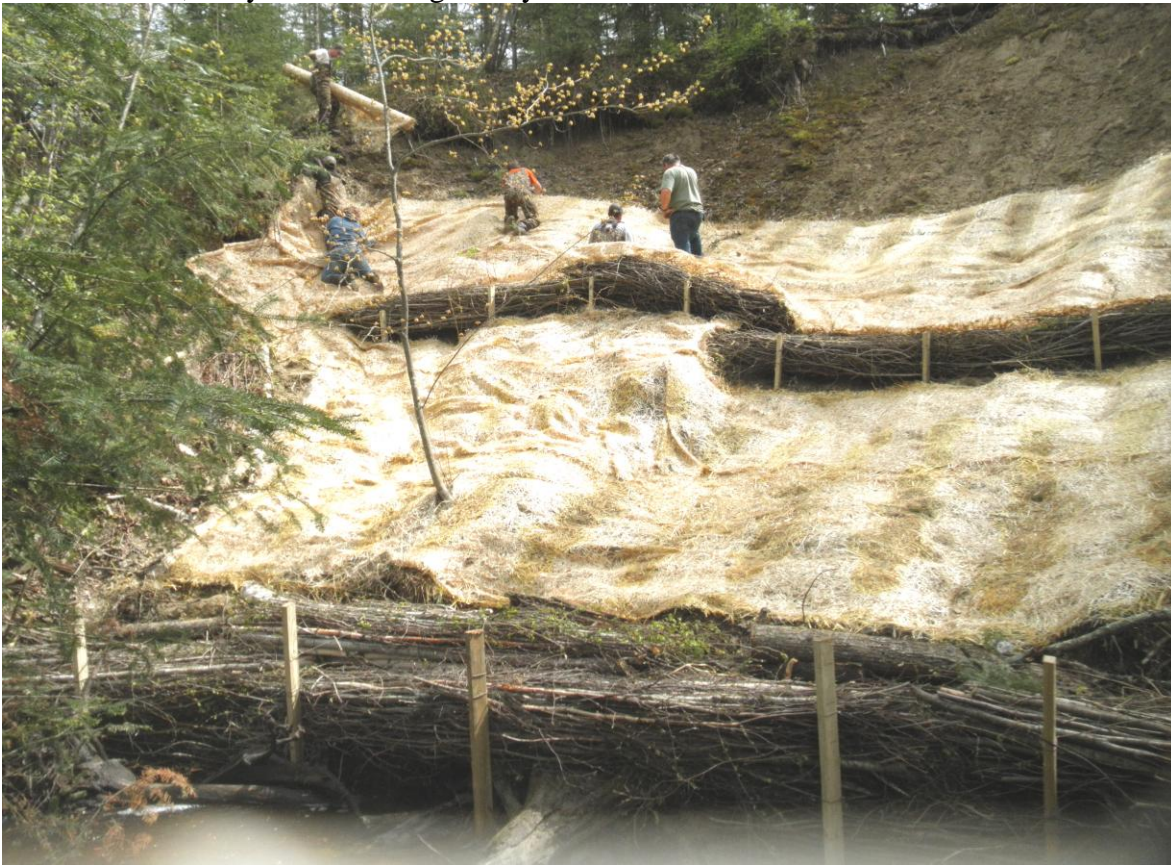
Installation of brush bundles and erosion control blanket by SWCD on May 9 th .
